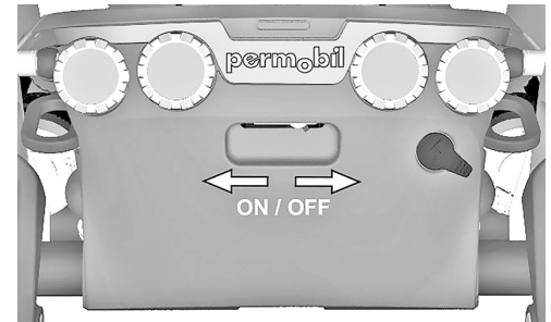
Figure 200. Main circuit breaker located under the Permobil logotype on the rear cover.
