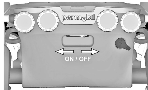
Figure 223. Main circuit breaker.
