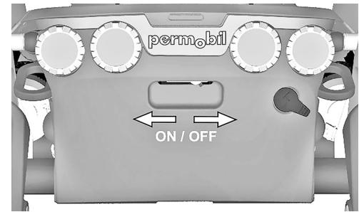
Figure 180. Main circuit breaker.
